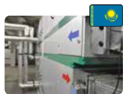
Air-conditioning, Public Hall, Astana, Kazakhstan
