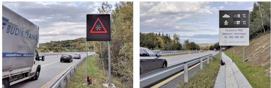
Fig. Foxtrot systems also work continuously and control information boards displaying the air temperature 1 and the road surface temperature along the sixth section of the highway and also on two warning traffic signs (PDZ) which display weather information. Photo by: Vit Jadrnicek
