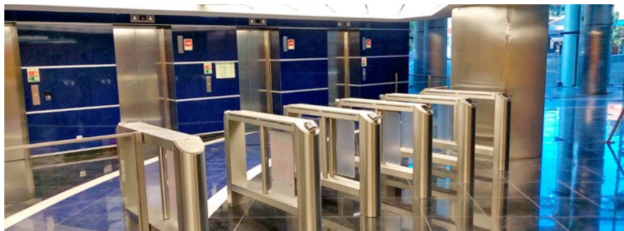
Fig. Entry turnstiles are the base of the bank access system.
