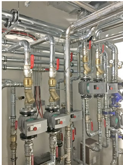
Fig. Heating and cooling circuits before insulations; two heat pumps, two large accumulation tanks, air compressor, central recuperation unit and two wide fields of the control system cabinets and high-voltage circuits were placed in the energy-centre (energocentrum); source: Teco, a. s.
