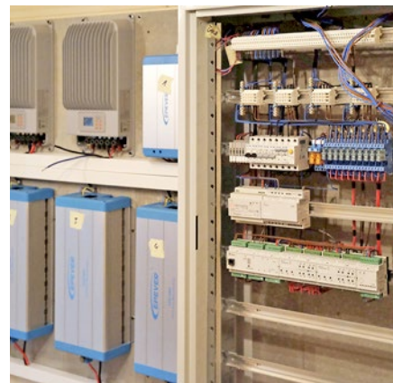
Fig. A distribution cabinet with Foxtrot located in the electrical room. On the wall you may see charging modules and inverters powered by batteries.
