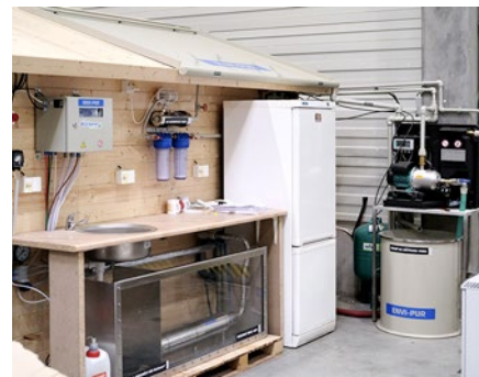
Fig. Testing assembly in a warehouse hall. The inner garden house dimensions match exactly the size of the future engineering room. The equipment for the island house – refrigerator, water treatment, water heating, waste system including water filtering plant are located outside of the house.
