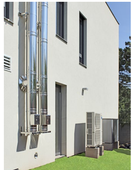
Fig. The outdoor unit of the heat pump is located in front of the house on the south. Chimney units on the façade are led from the bivalent source which is switched on when the surrounding temperature falls down to a minimum.
