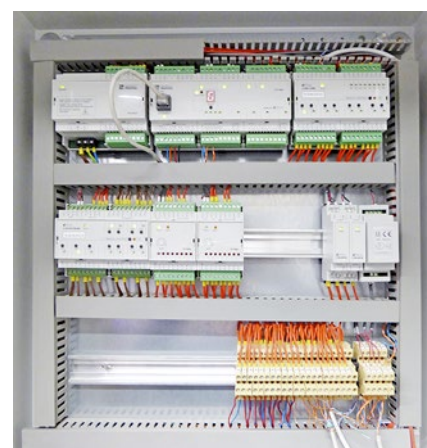
Fig. Cabinet with Foxtrot installed in VIPAX.
