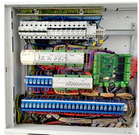
Fig. 1. View into the Smart Control system cabinet that is being developed and supplied by TENAUR s.r.o. On the right you see the OEM version of Foxtrot in "Open Frame" and a specially arranged input and output configuration that are used to control the heat pump. It is combined with standard expansion modules.
