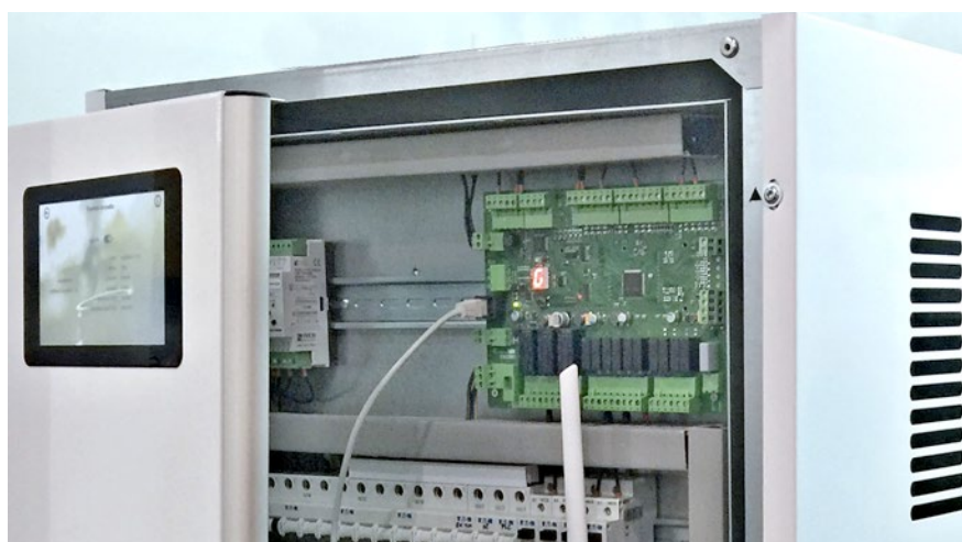
Fig. At Aquatherm Prague fair we had a look under Energybox cover. Behind the display there is placed Foxtrot in OEM version CP-1970.
