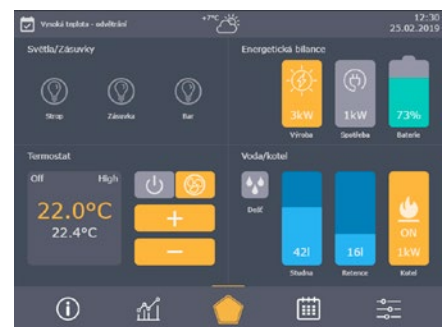
Fig. Control screen developed for the control and monitoring of the Czech self-sufficient house project.
