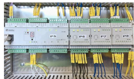
Fig. Basic module and 3 expansion modules handle the entire control of the hydro power plant
