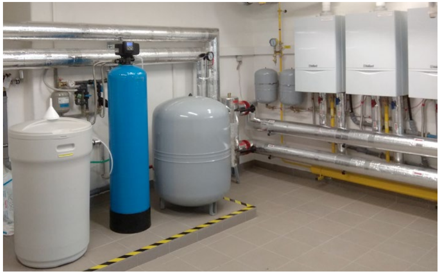
Fig. This picture shows the central source of heat together with a cascade of gas boilers
