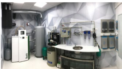
Fig. A unique show room equipped with Foxtrot which controls the technologies of the island house – a house which is not connected to the public power grid. This house may be seen in Prague at the ELPRAMO company headquarters.
