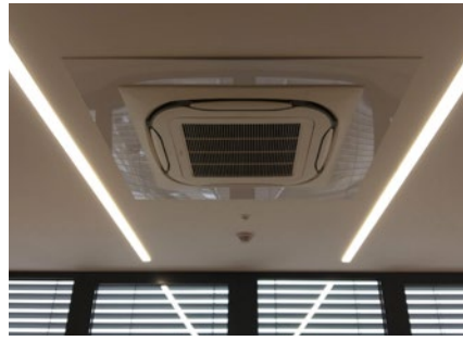
Fig. 4 Blinds, light fixtures, cooling and heating systems, ventilation and the access system represent one integrated and logically operating unit installed in each office and controlled by Foxtrot
