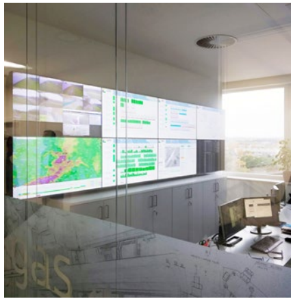
Fig. GEEN monitoring center in the reconstructed upper floors of the high-rise building at Mariánské náměstí in Brno. Here we can also “monitor” the entire city of Brno.
