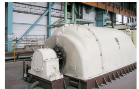
Fig. Steam turbine at Martinská teplárenská a.s. controlled by Tecomat NS 950
