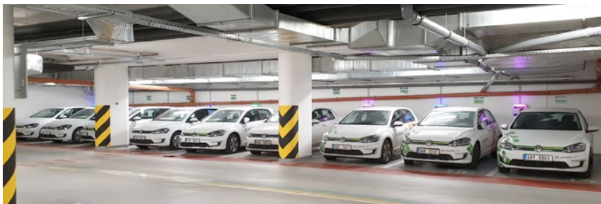
Fig. 6. Parallel recharging process of the entire fleet of e-Golf vehicles is fully controlled by Foxtrot
