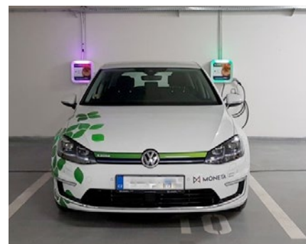
Fig. 3 Each parking space in the underground parking lot in Moneta bank is equipped with a recharging cable. The status of the recharging box is indicated by color LED indicator. All recharging stations are connected with two-wire CIB installation bus and are monitored online by Foxtrot using 150 ms clock tact. The current 36 parking spaces, each equipped with a recharging station, will be expanded in the near future to reach 100 spaces.
