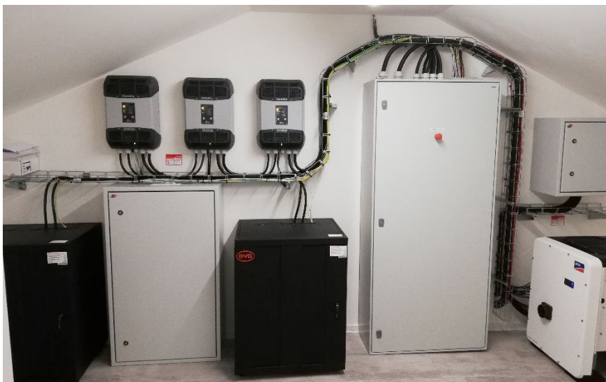
Fig. Picture showing the installation of a 3-phase hybrid power plant in Jimi Tore s.r.o.
