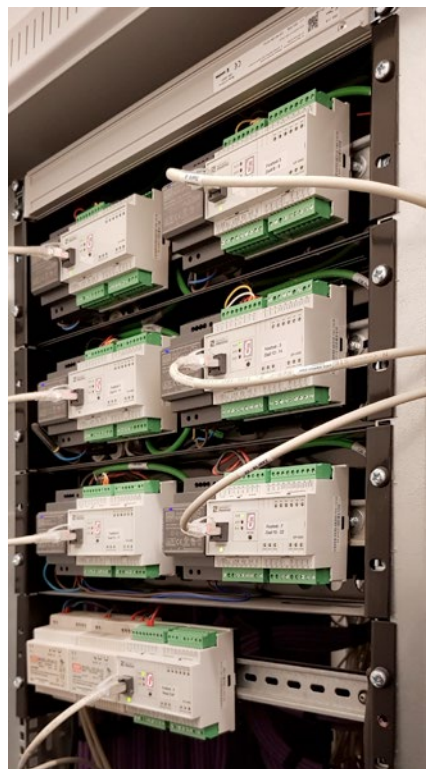
Fig. Seven basic Foxtrot modules CP-1005 are the backbone of the control infrastructure which monitors the congress halls.
