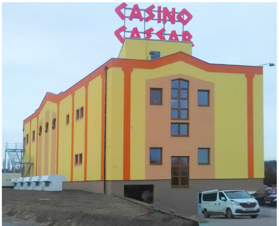
Fig. CASINO CAESAR – on the left: a cascade of five “air-water” heat pumps – 5x WPL57
