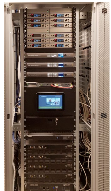
Fig. Distribution cabinet with multi-channel audio amplifiers, video matrixes and wireless microphones.
