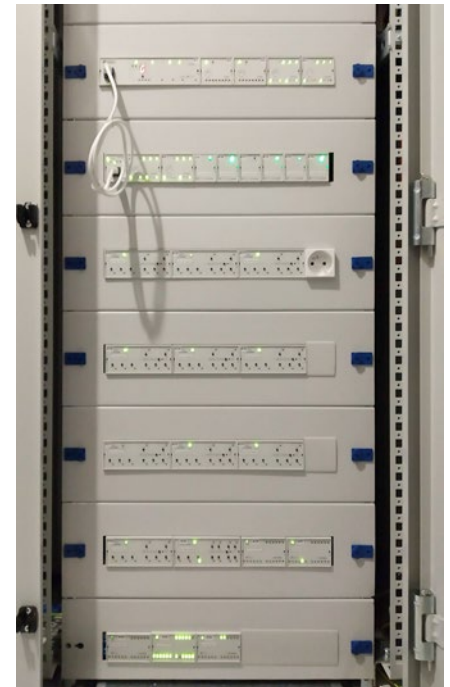
Fig. 8 This picture shows Foxtrot control system in the distribution cabinet which manages the entire floor. You may see ballasts for six branches of DALI buses. Other components are installed in rooms, such as sensors and switches, and are connected through CIB (Common Installation Bus™)
